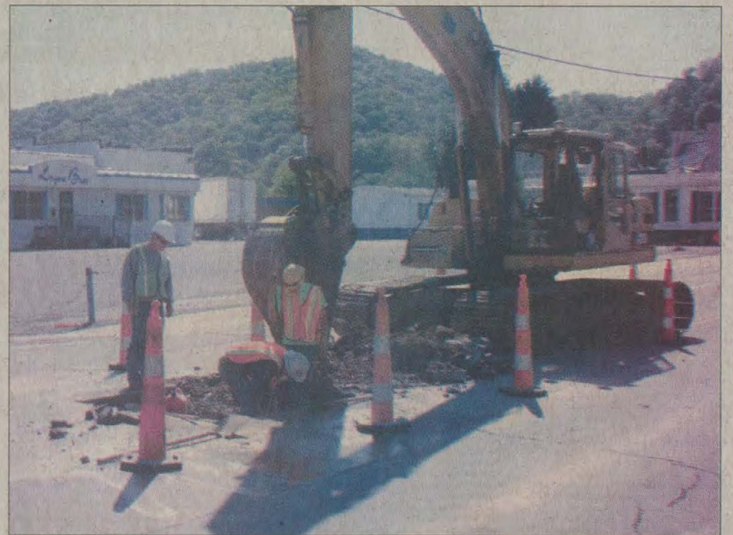
Photo by Devin Clifton Road crews were hard at work in Prestonsburg this week on various projects, including this one on South Lake Drive.
