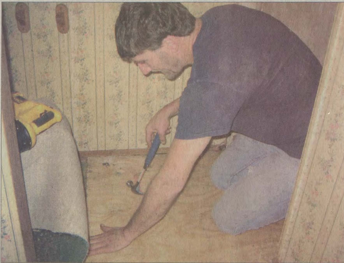
Workers with the Big Sandy Area Community Action Program weatherization crew recently completed work on a Printer home, replacing skirting and floors and installing a new heat pump, floor insulation, smoke and carbon monoxide detectors, window caulking and two new doors.
