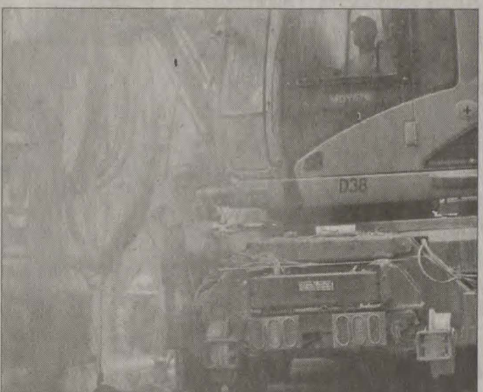
A typical drilling operation makes necessitates closing the road to all traffic. The drilling rig itself takes up almost two lanes. It takes about 10 minutes to drill one hole and place a length of railroad steel inside.
