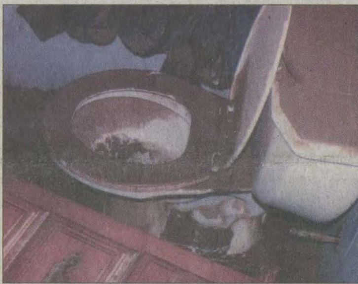
This photo taken by William Ward after the floodwaters receded show the levels of the water which overtook the entire bathroom of his and his wife's trailer between the Twin Bridges at Martin during the hard rains and flooding in the first week of May.
