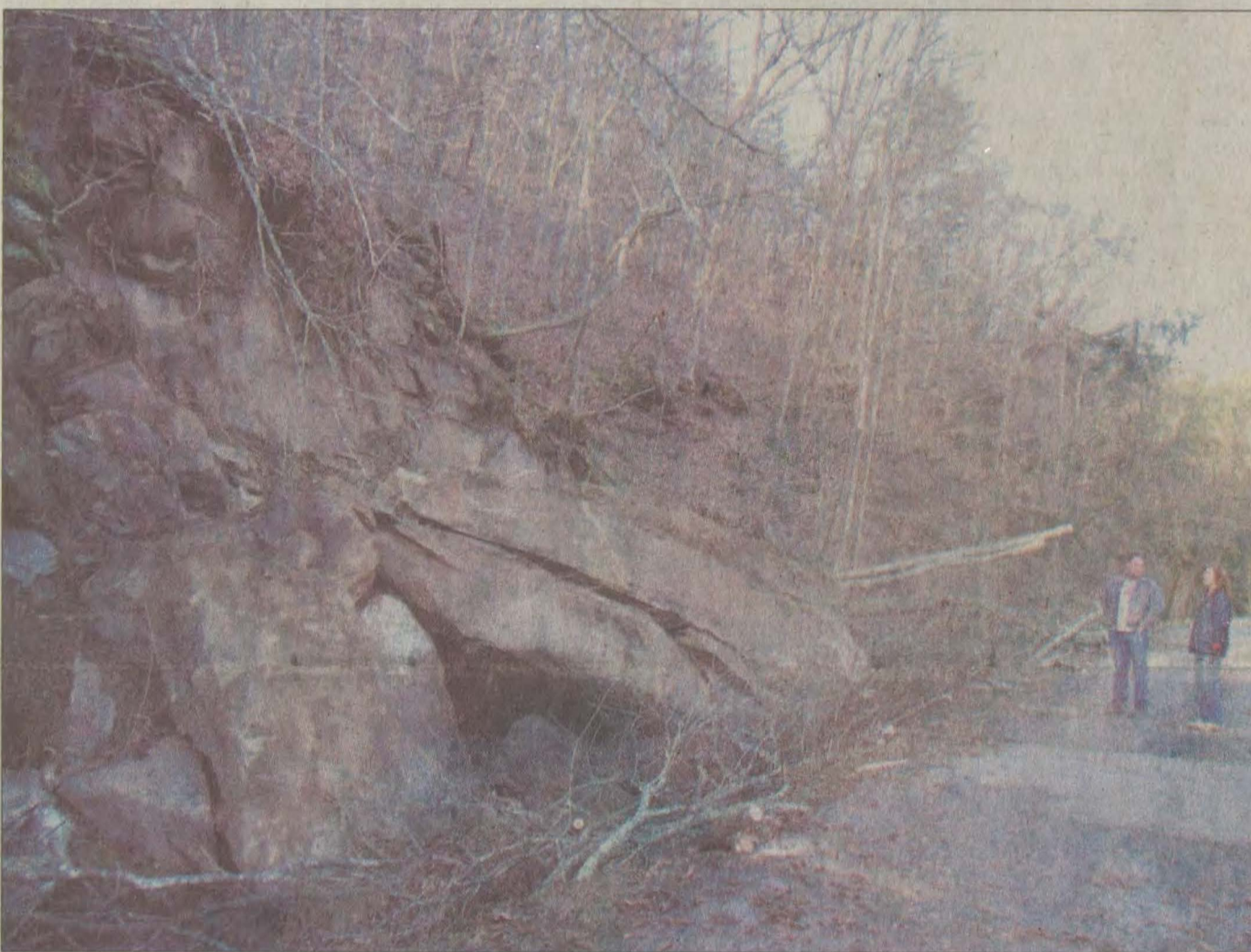
An early morning rockslide along the Left Fork of Little Paint resulted in minor property damage Friday, but had county officials working through the day to clear the road.
