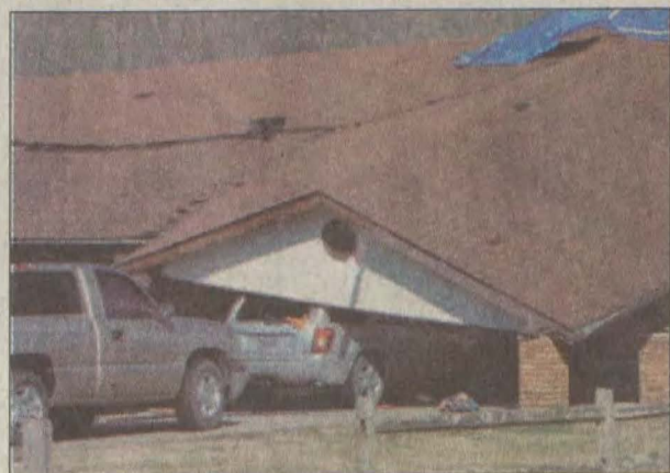
This carport collapsed in the wake of 70 mile an hour winds during Wednesday's storm.
