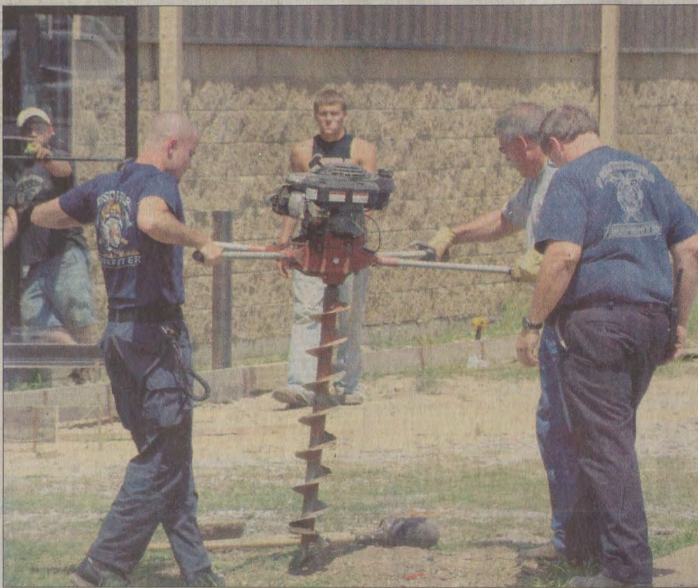
The Prestonsburg Fire Department and members of Prestonsburg City Utilities were called out Friday afternoon when crews working at the new West Virginia Electric Supply building drilled into a gas line.
