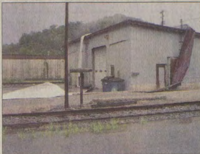
Power lines weren't the only thing affected by Tuesday's storm. High winds blew away the roof of this building in West Prestonsburg, across from Action Petroleum.
