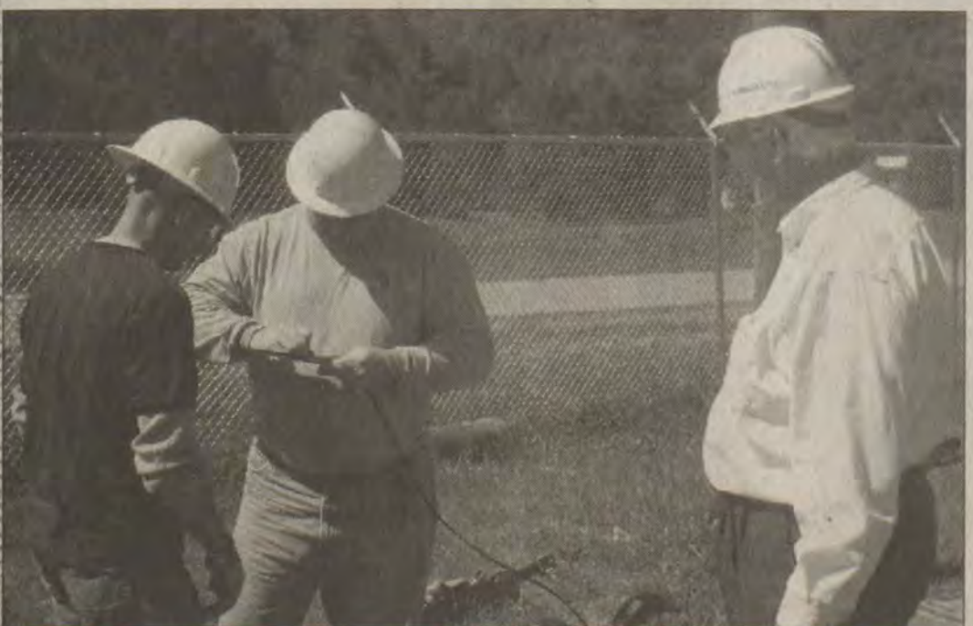
Tom Charles, right, an instructor with Big Sandy Community and Technical College, watches as Gearheart Communications employees, from left, Chris Rose and Donnie Ray prepare to participate in pole climbing training at the college's "pole climbing farm" at Betsy Layne. A training collaboration between the college, Eastern Kentucky Concentrated Employment Program, Inc. (EKCEP), and Big Sandy Area Community Action Program brought this and a vast array of other essential employee training to Gearheart's telecommunications companies at little or no cost to them.
