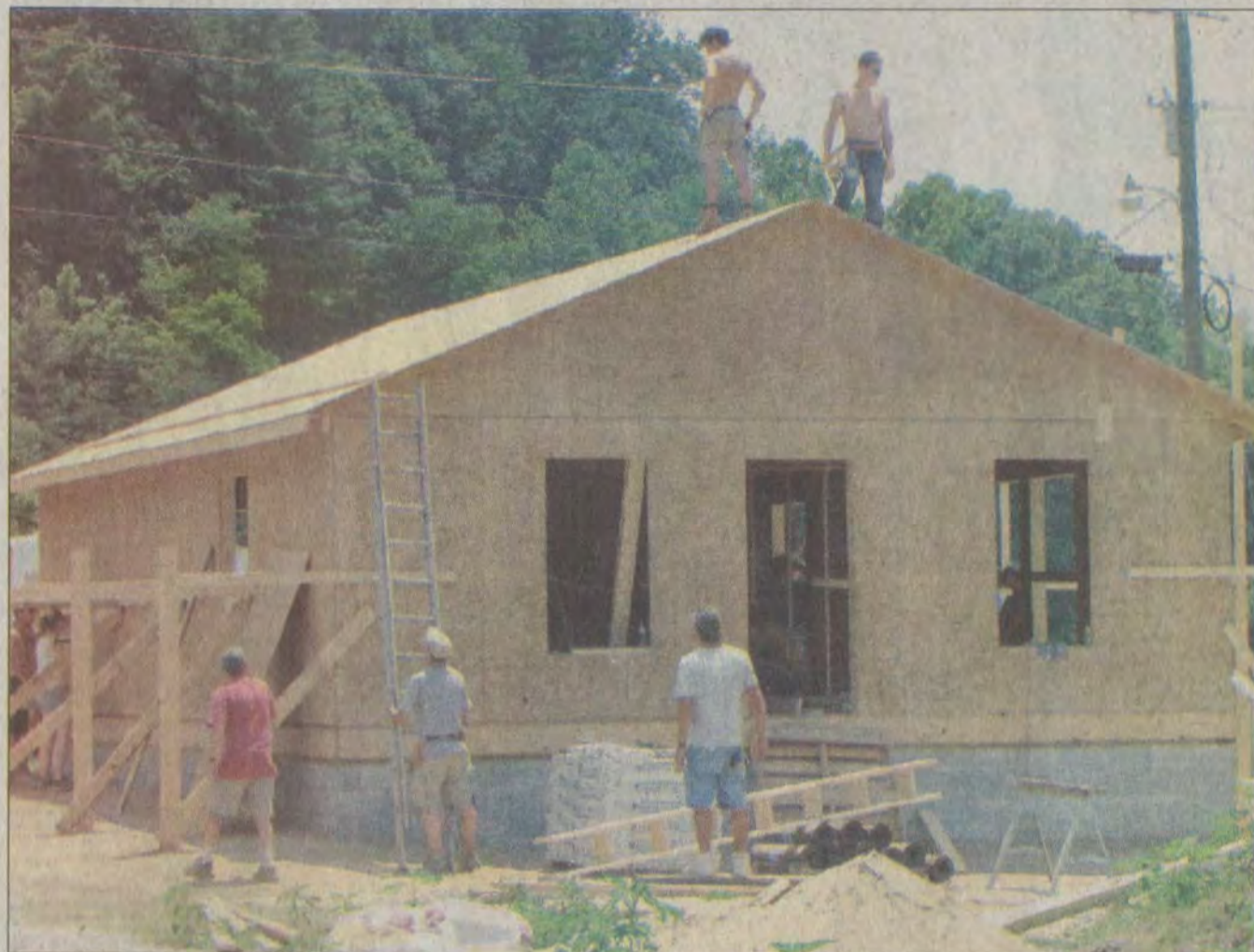
Members of the United Churches of Durham, Conn., have made the 12-hour trip to Eastern Kentucky the last six years to construct homes as part of the LINKS program.
