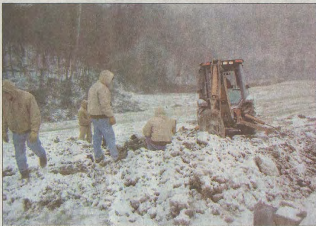
A city utilities crew worked to replace a water pipe on Abbott Mountain that burst early Wednesday morning.
