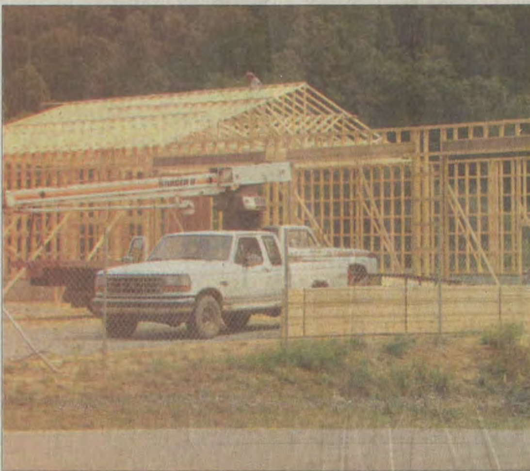
Crews began construction on the new Middle Creek Volunteer Fire Department a few weeks ago. The new building is located just past Park Place Apartments on Route 114.
