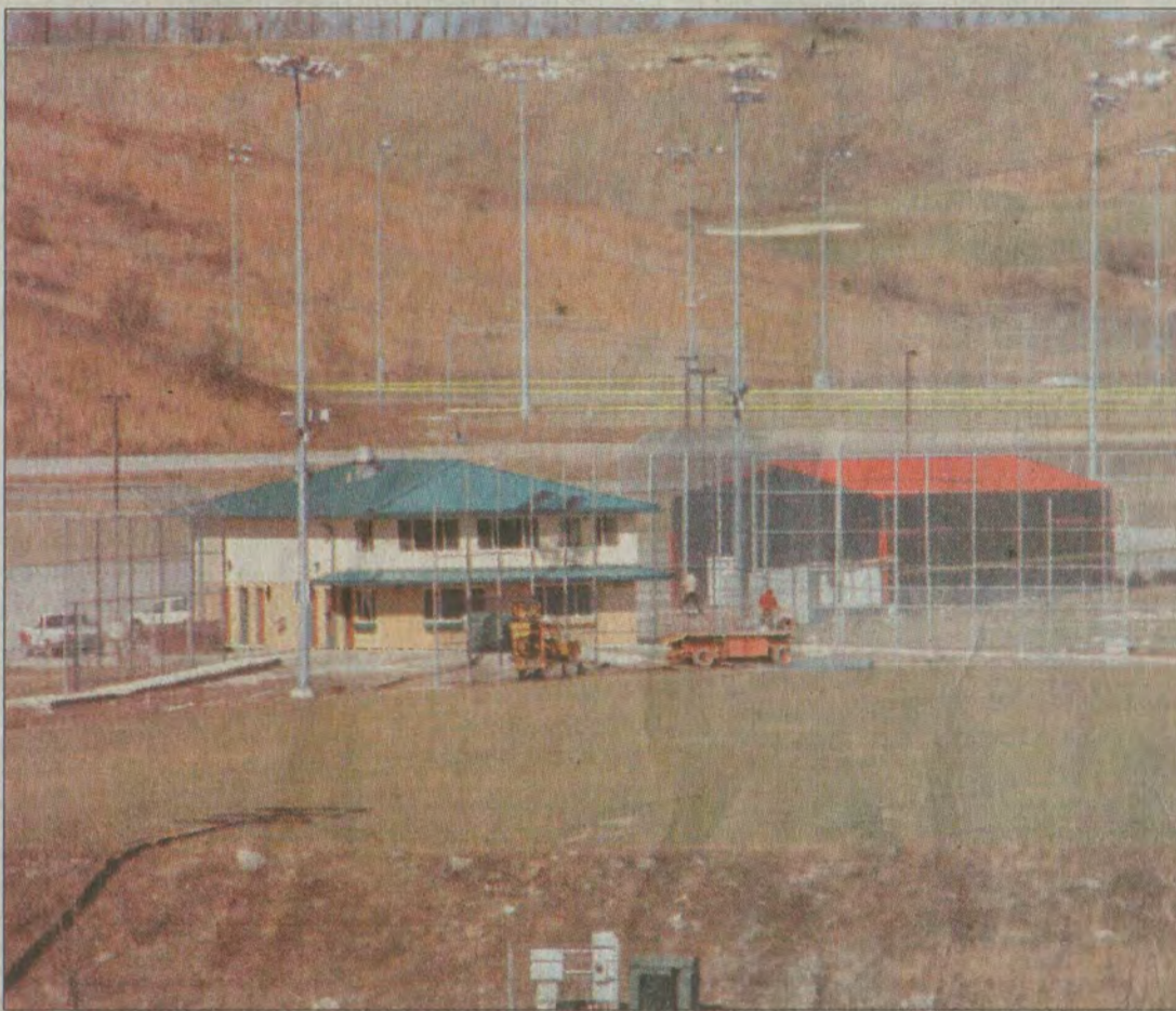
City workers continue to work on the new Prestonsburg SportsPark located at Stonecrest. Finishing touches are being added daily.
