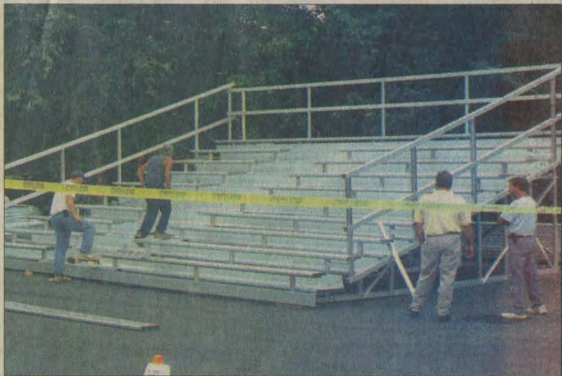
Mayor Jerry Fannin observed the progress of the new bleachers being erected Thursday for the "Fridays Alive" concert series in downtown Prestonsburg.
