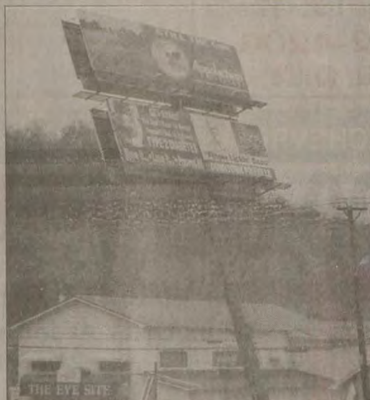
Friday's storm damaged a UNISIGN billboard on US 23 at Coal Run, forcing evacuation of the Eye Site building. "At first we thought the power would have to be turned off in order to remove the signs and the post they are mounted on," said Frank Castle, Maintenance Engineer of Highway District 12. "That would have meant that all the traffic signals through Weddington Plaza and Weddington Square would have shut down. Thankfully, the folks from UNISIGN used a different approach to the problem and we didn't have to turn off the traffic signals."
