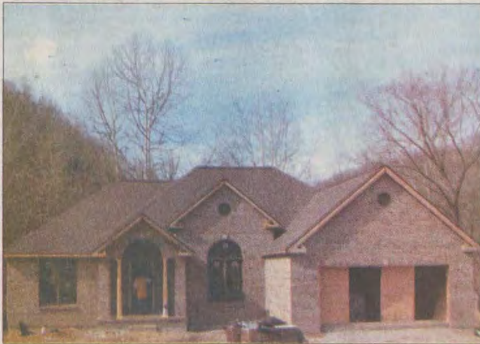
This home, located in the Cross Creek II subdivision, at Staffordsville, is in its final stages of completion. The home is a project of students from Big Sandy Community and Technical College and will be available for sale to the general public in the months to come.
