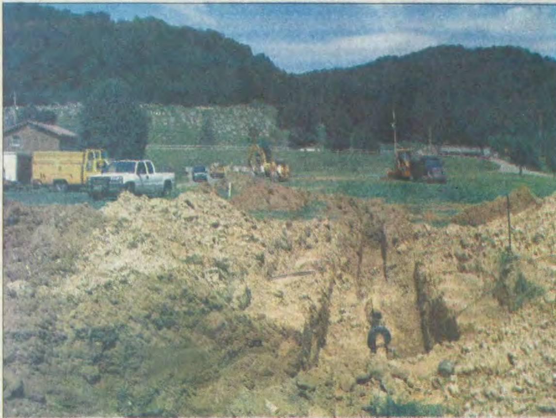
MarkWest's decision to replace a gas pipeline at the site of an explosion last year has left some Ivel residents nervous. The work is supposed to finished this week.
