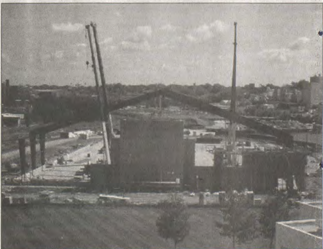
Construction on the University of Louisville's new Trager Indoor Practice Facility, located just north of Papa John's Cardinal Stadium is well underway.
