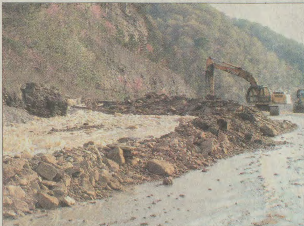
More than two dozen state highway workers constructed this earthen berm to prevent further water damage to Route 80.
