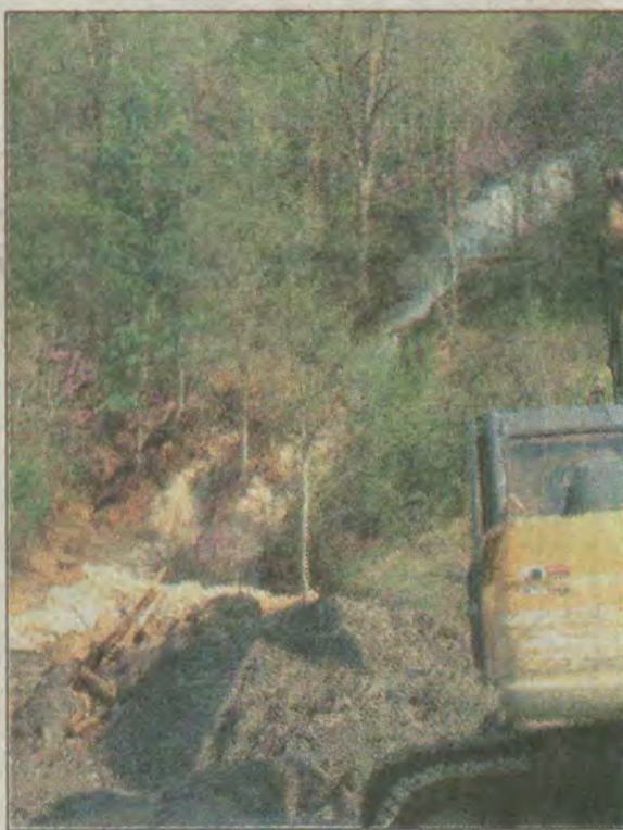
Water is still flowing steadily off the hillside above the road, a Transportation Cabinet engineer said yesterday. Officials can't determine how extensive the damage is until the water subsides.
