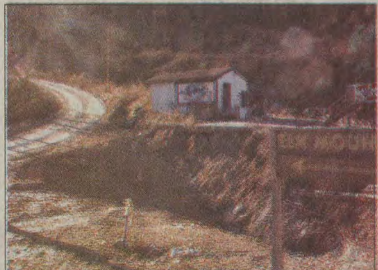
photo by Mary Music Residents are wondering why this gaping hole on Rt. 302 has not been fixed. It washed out during the Memorial Day flooding last year and is still on a waiting list for repairs.
