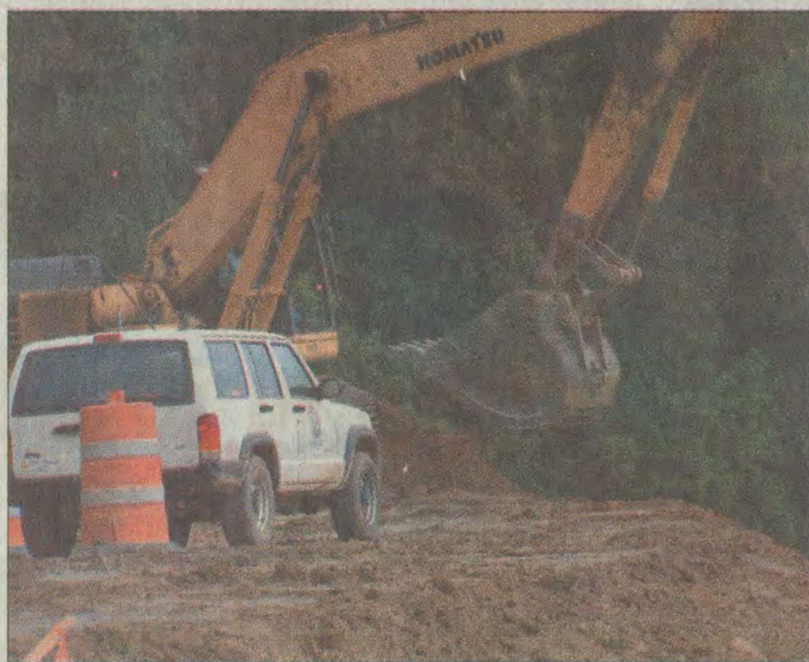
Construction continues on University Drive. Road crews last week began channeling the shoulder of the road near the Big Sandy Community and Technical College entrance. This area will be filled in, Department of Transportation workers said, in order to expand the width of the road. Construction on the project, which began in April, is expected to last until winter.
