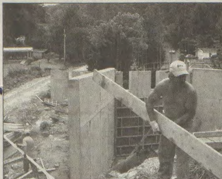
photo by Mary Music Eric Hamilton, forefront, and Manuel "Hershey" Adams worked Wednesday on building a new bridge on Ray Branch at Middle Creek.
