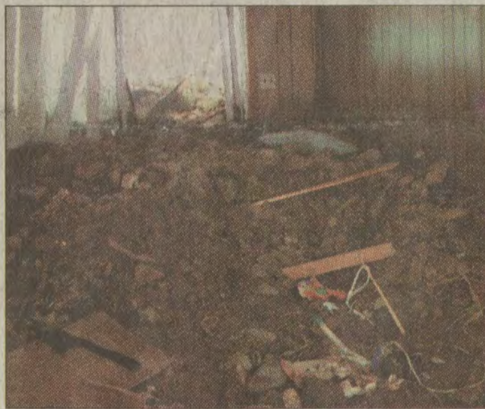
The Hales were asleep in their bedroom when the Memorial Day flood washed rocks and mud into the home, several feet deep in some spots. The couple barely made it out alive.
