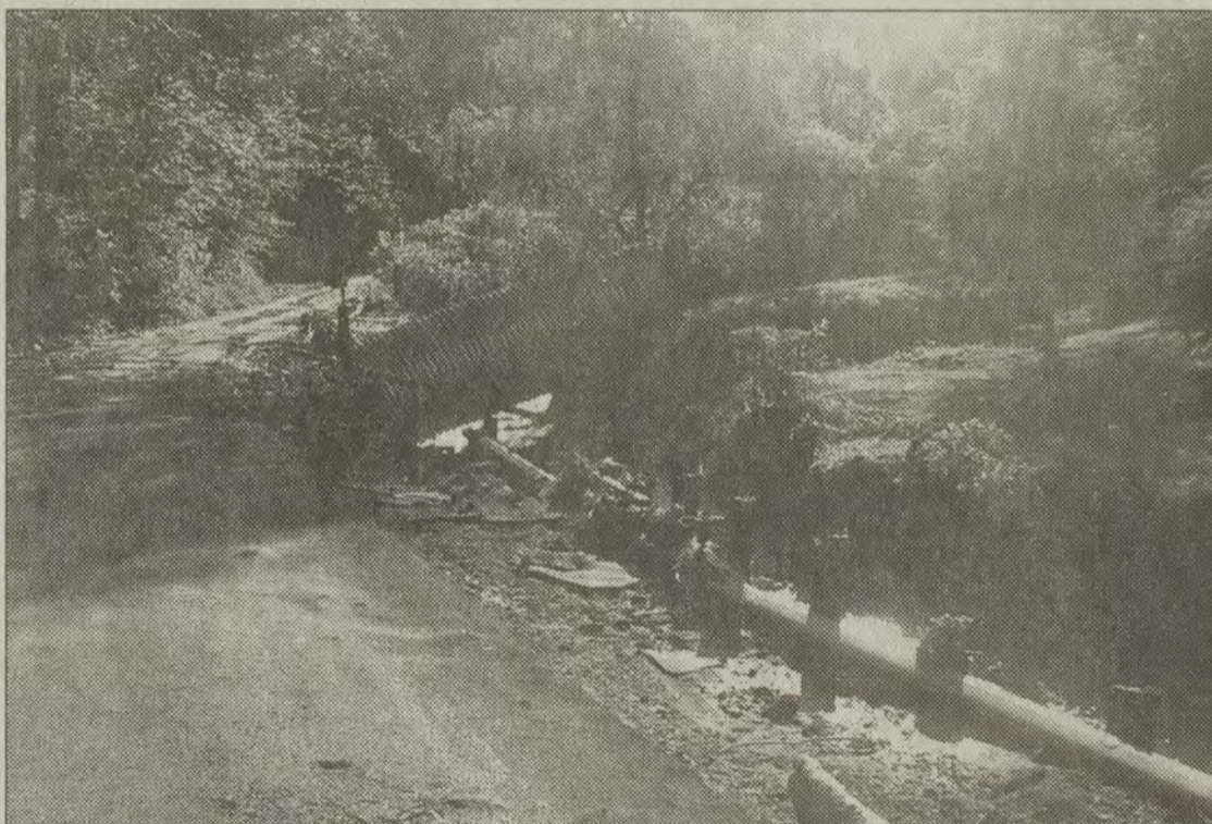
photo by Joy Baldrige Countless culverts across Floyd County were damaged or, as in the case of this one at Rough and Tough, completely swept away by flash flooding.
