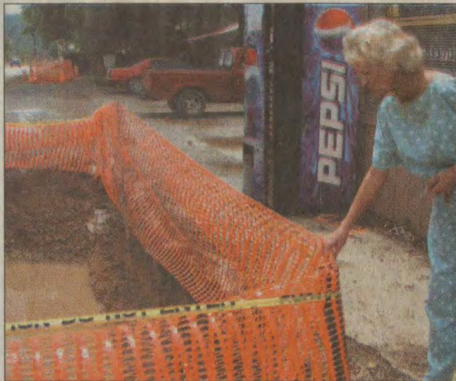
With complaints mounting from area businesses regarding the current construction on University Drive, business owner Barbara Slone is throwing another complaint on the pile. Slone, who operates the Big Sandy DUI Program, offering classes to individuals charged with driving under the influence, says this 10-foot-deep hole located approximately two feet from the entrance of her establishment is driving customers away and presenting a noticeable danger to those who do come. "I'm ready to close down," Slone said. "They're killing me." A similar hole sits unfilled a few feet away, in front of the Neeley apartment complex.
