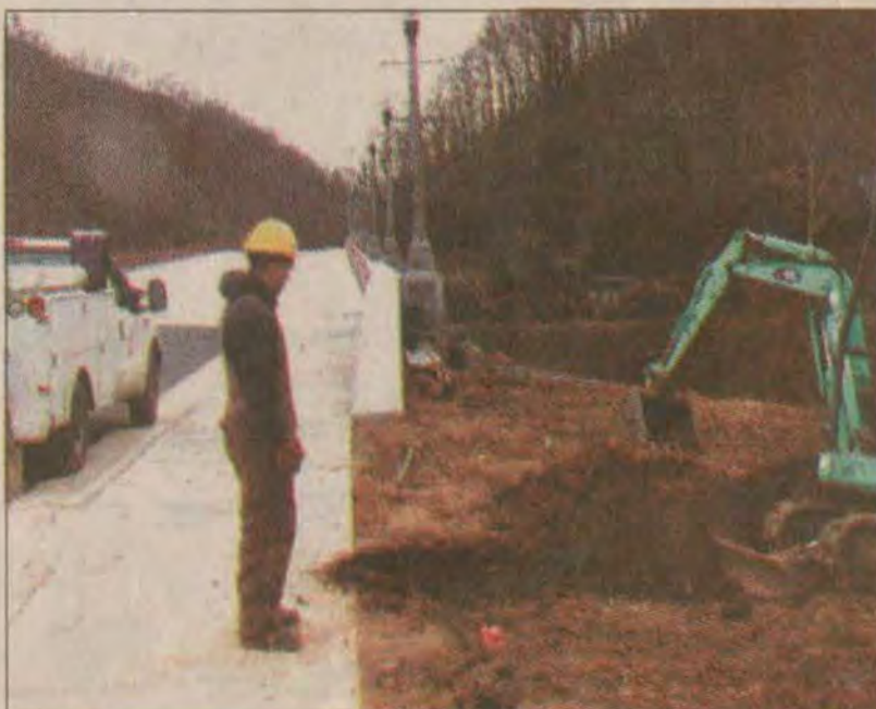
Dudley Craycraft, a laborer with the Kentucky Highway Department, and foreman Eric Justice, not pic- tured, dug trenches Tuesday to run electrical supply to the light posts on the new Town Branch Bridge. The bridge official- ly opened to traffic Thursday.
