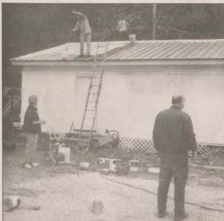
Students from the Perkins Job Corps Center carpentry and maintenance departments observed National Make a Difference Day by working with the Johnson County Road Department at the Johnson County Park. The students were supervised by Dennis Conley, shown in photo, and Roy Picklesimer.
