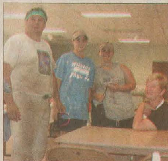
A group of 76 people from Presbyterian churches on the south side of Chicago are working with Doreen Martin, of Drift Presbyterian Church, by supplying and labor to help Floyd County residents who have homes in need of repair.
