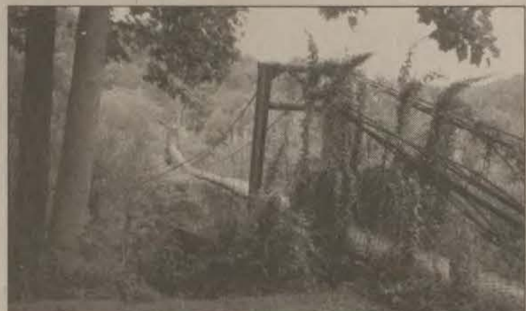
The pedestrian bridge that spanned Levisa Fork, at River, was originally built by the River United Methodist Church and was beyond repair.
