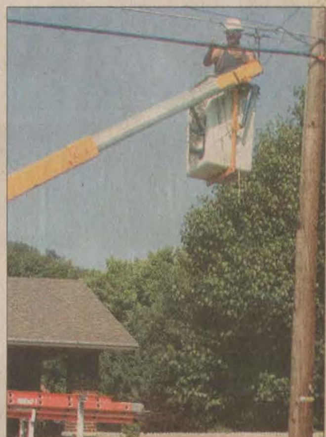
Ruben Macais, of Cable Crafters Construction, was splicing an upgraded fiber optic cable that Charter Communications will be activating.
