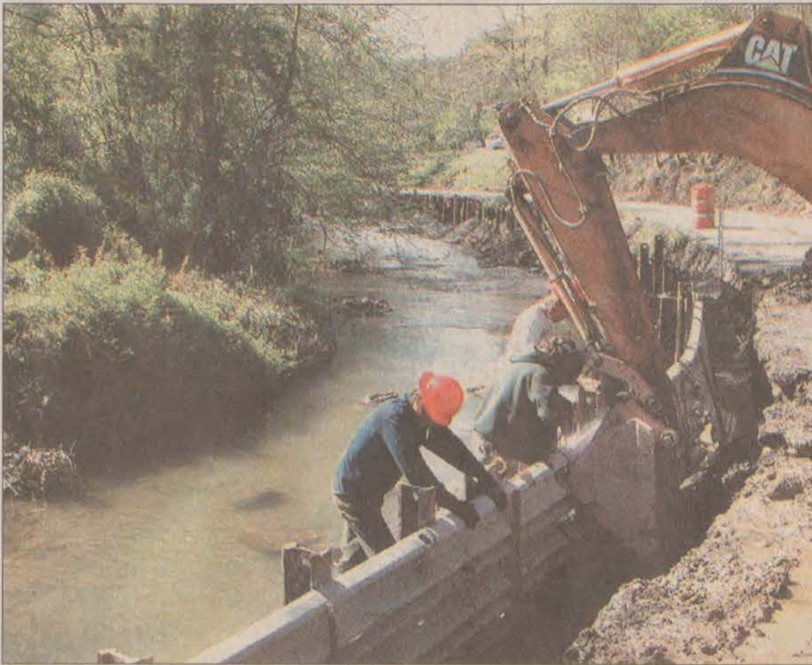
Route 3379 at Branham's Creek was closed Friday and Saturday and will be closed next Saturday and Sunday as work crews replace pipes along the route. Robin Trimble Justice, resident engineer with Department of Highways District 12 in Pikeville, said motorists should use alternate routes in and out of the area.
