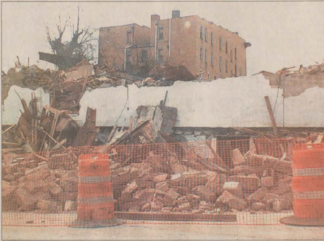
Sections of Jackson looked more like war-battered Afghanistan Monday morning after work began to clear room for a new justice center and jail. The demolition was not without its problems, however, as a wall from one building knocked out power and telephone lines, leaving many residents in the dark.
