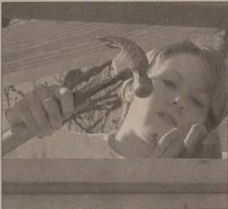
Workfest 2002 will host close to 500 college youth during Spring Break this year. The annual event, sponsored by the Christian Appalachian Project, will repair dilapidated homes for needy families in Appalachia during the weeks March 4-8 and 11-15, 7 a.m. to 4:30 p.m. daily and 7 to 10 p.m. each evening.
