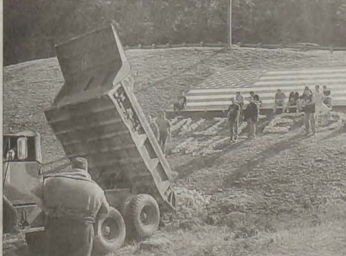
Students from Opportunities Unlimited paused in their work to watch as another load of large rock was deposited at the entrance intersection to the town of Martin.
