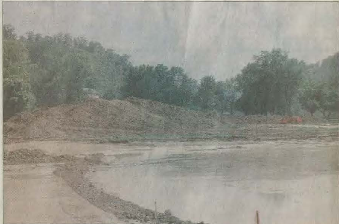
Work on the long-awaited East Kentucky Center for Science, Mathematics and Technology has taken a more visible turn, as work crews have begun site preparation in recent weeks. Tons of dirt have been hauled in to raise the site out of the floodplain.
