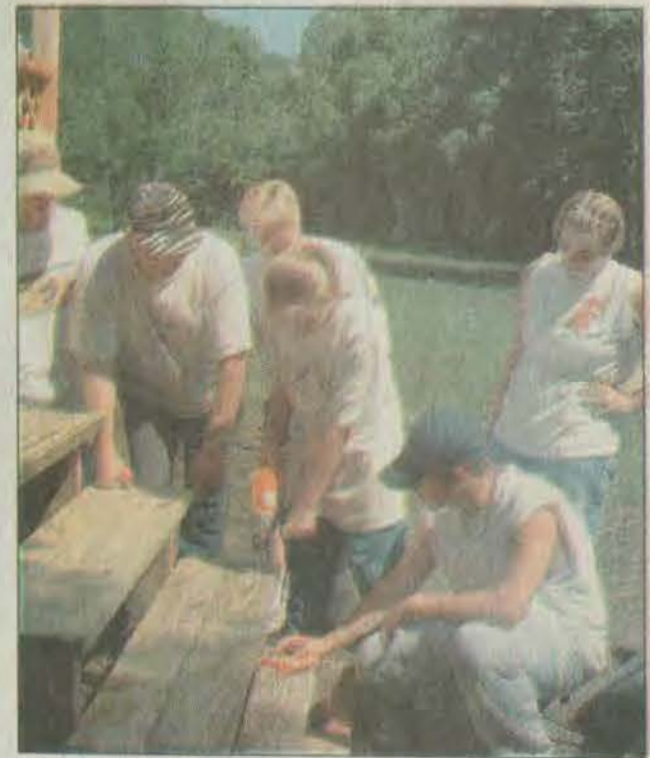
ASW volunteers worked in the hot sun on Wednesday, replacing the steps to the home of John and Juanita Hamilton, whose property was severely damaged by flooding last week.
