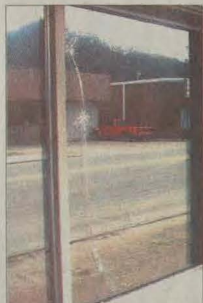
A splintered crack winding along the Wilson, Sowards, Polites and McQueen law office window on South Lake Drive in Prestonsburg stands as the result of a deer colliding with the law office window this past Friday.
