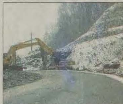
Work crews from Tabb Construction returned to the job to assist in the waterline replacement after being scheduled a weekend break due to winter weather.
