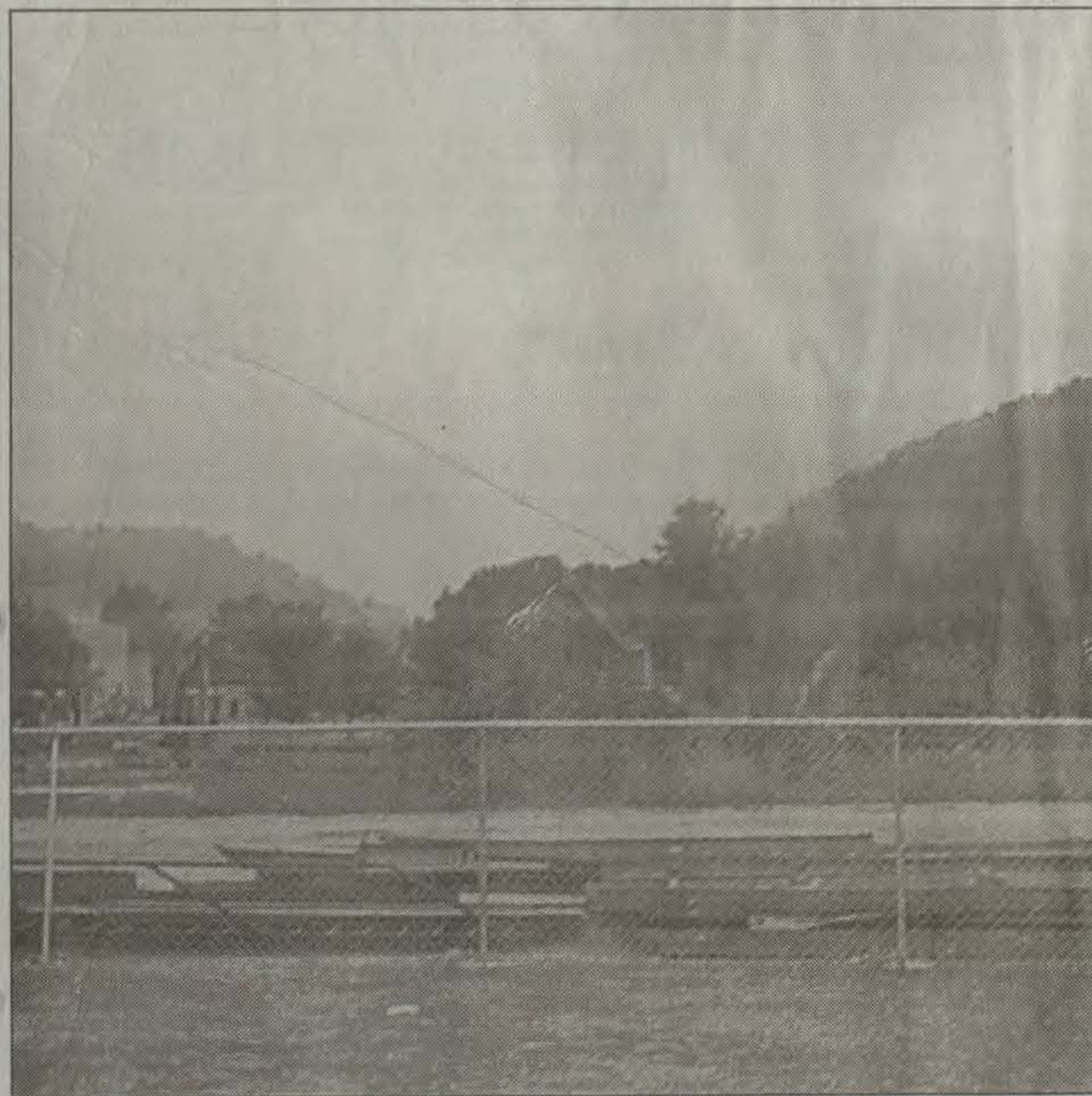
Construction workers clean up the remains of the Martin Student Center which was recently razed in order to make room for a new building. (photo by Willie Elliott)
