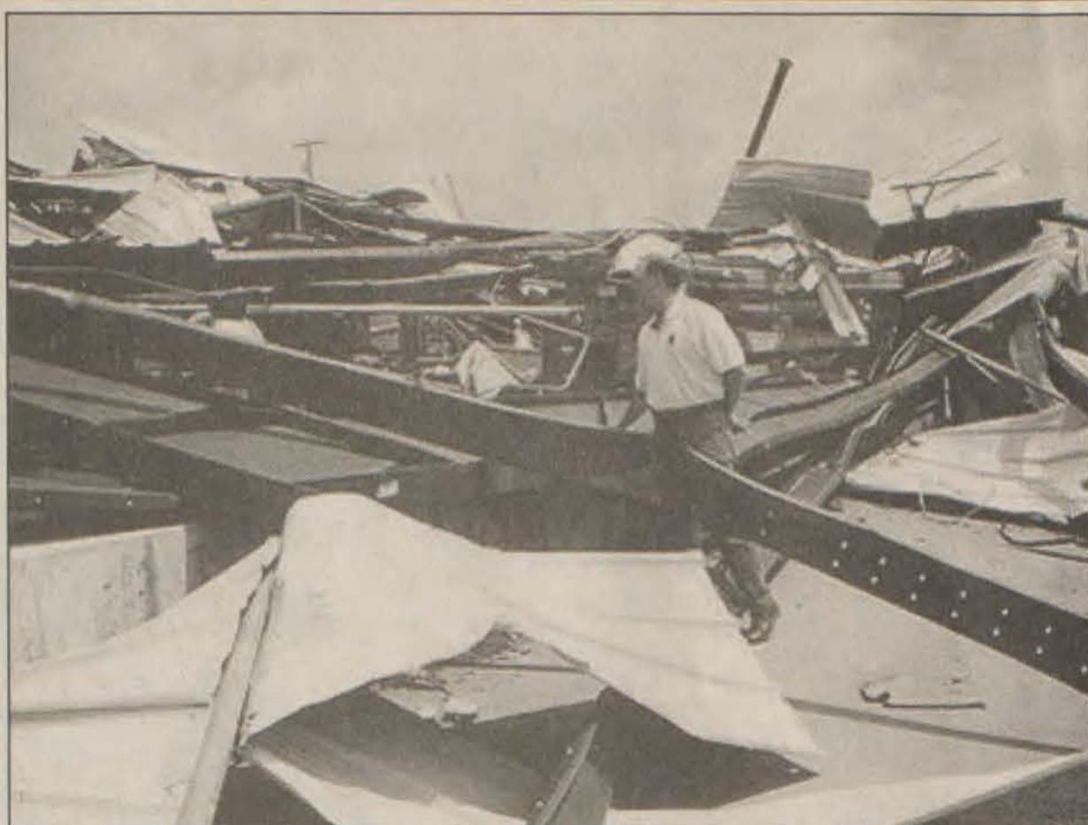
Lt. Gov. Steve Henry looks at what used to be the sawmill area of Baillie Lumber in Leitchfield. Eight employees survived inside the twisted and flattened building.
