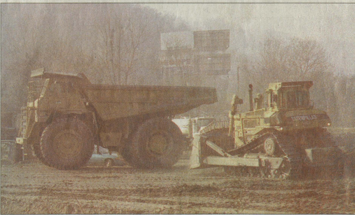
The road widening project on KY 114 near Prestonsburg Village can be slow going sometimes as workers take the mountain down to make room for the another two lanes. These two large machines are taking part in the earth removal and relocation. (photo by Willie Elliott)
