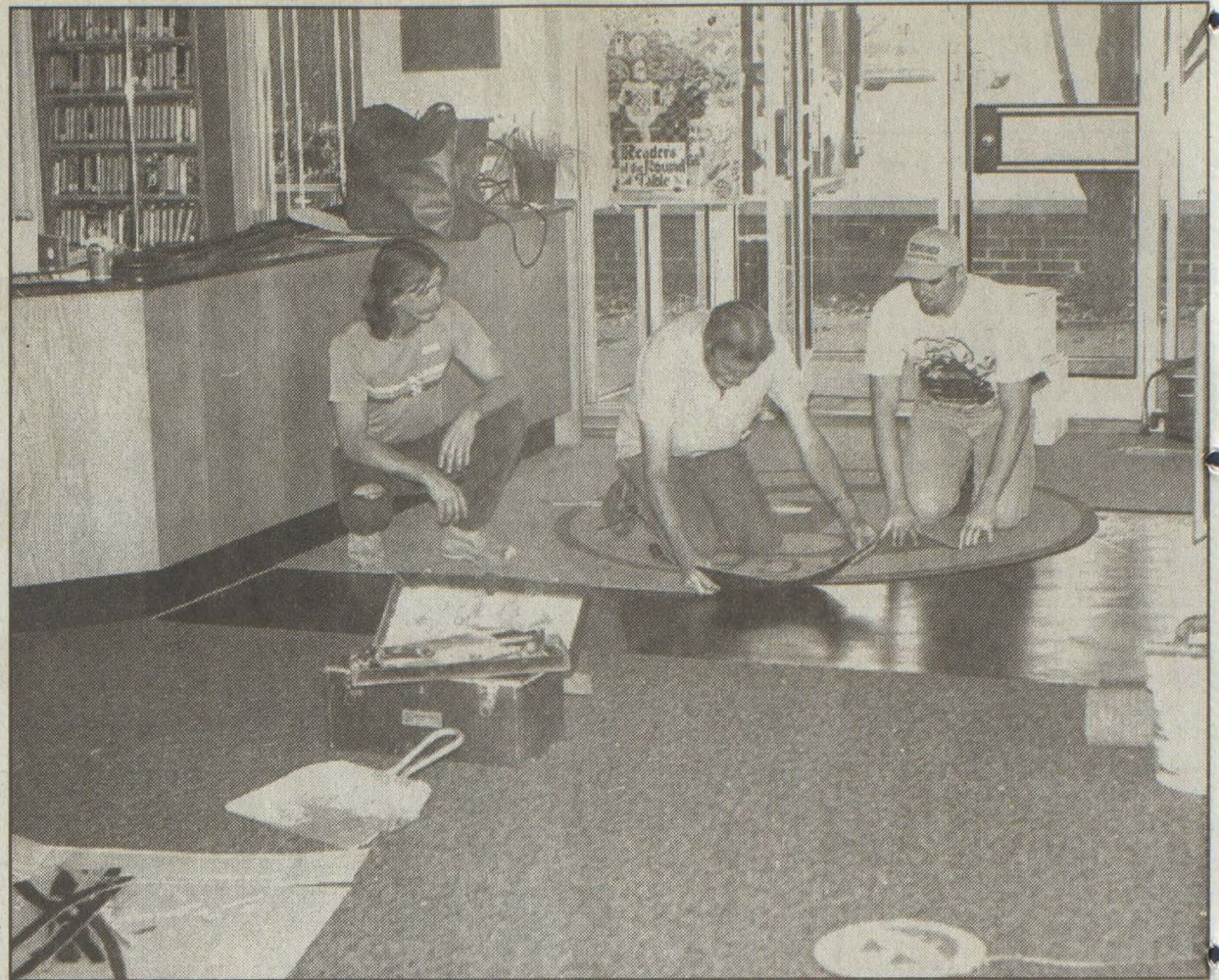
Patrons of the Floyd County Library can expect at least another week without services. The library has been closed since Nov. 1, as workers from Carpet Decorators install a new carpet. Especially catching is the carpet in the children's section. Carpet installers, from left, Rick Herdner, Tom Stansberry and Brian Stansberry were installing part of the carpet Monday morning. Patrons should also appreciate the carpet with the library's logo. The tentative date for completion is in time to open the library on Monday, Nov. 15. Library workers invite patrons in around the 20th of the month when the Christmas tree will be up. (photo by Willie Elliott)
