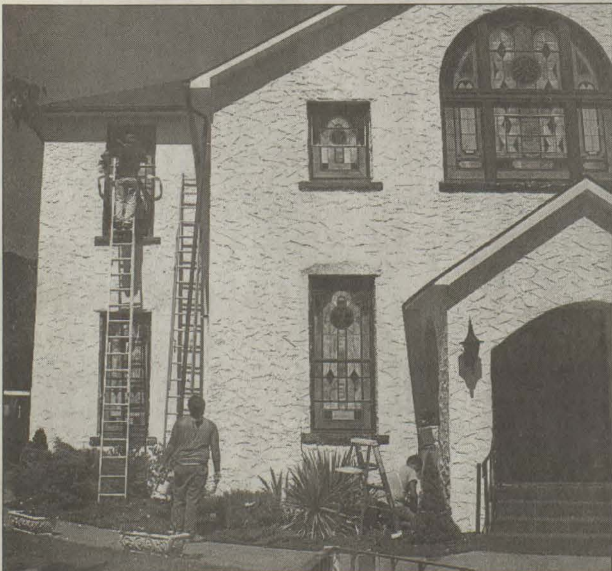
Workers apply a new coat of paint this week on the Third Avenue Freewill Baptist Church in Prestonsburg (which is located on South Central Avenue) as part of the spruce-up the church is receiving. (photo by Willie Elliott)
