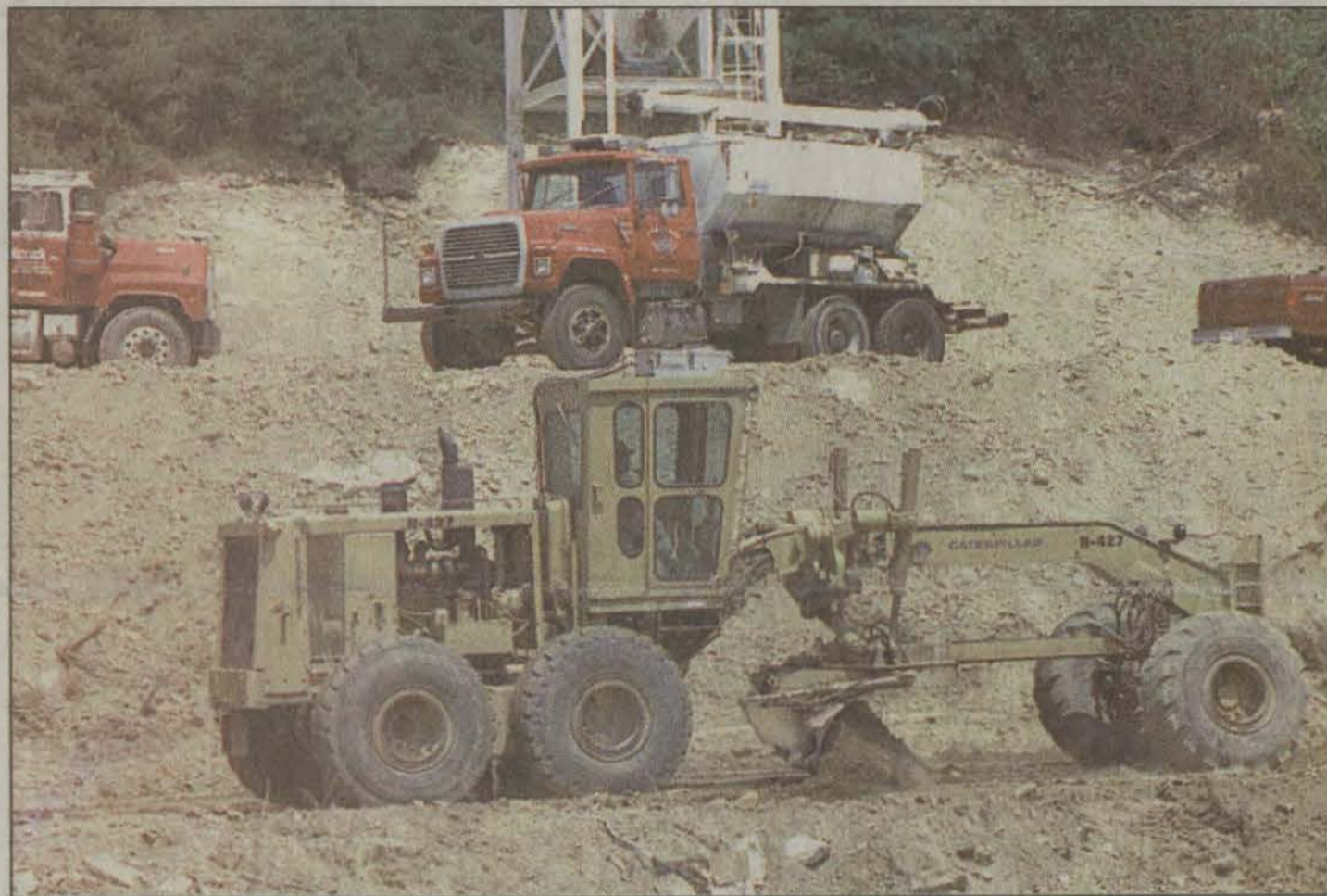
Construction work is underway on KY 114. Heavy equipment operators are building a four-lane highway that will make the Mountain Parkway a four-lane road into Prestonsburg. (photo by Ed Taylor)
