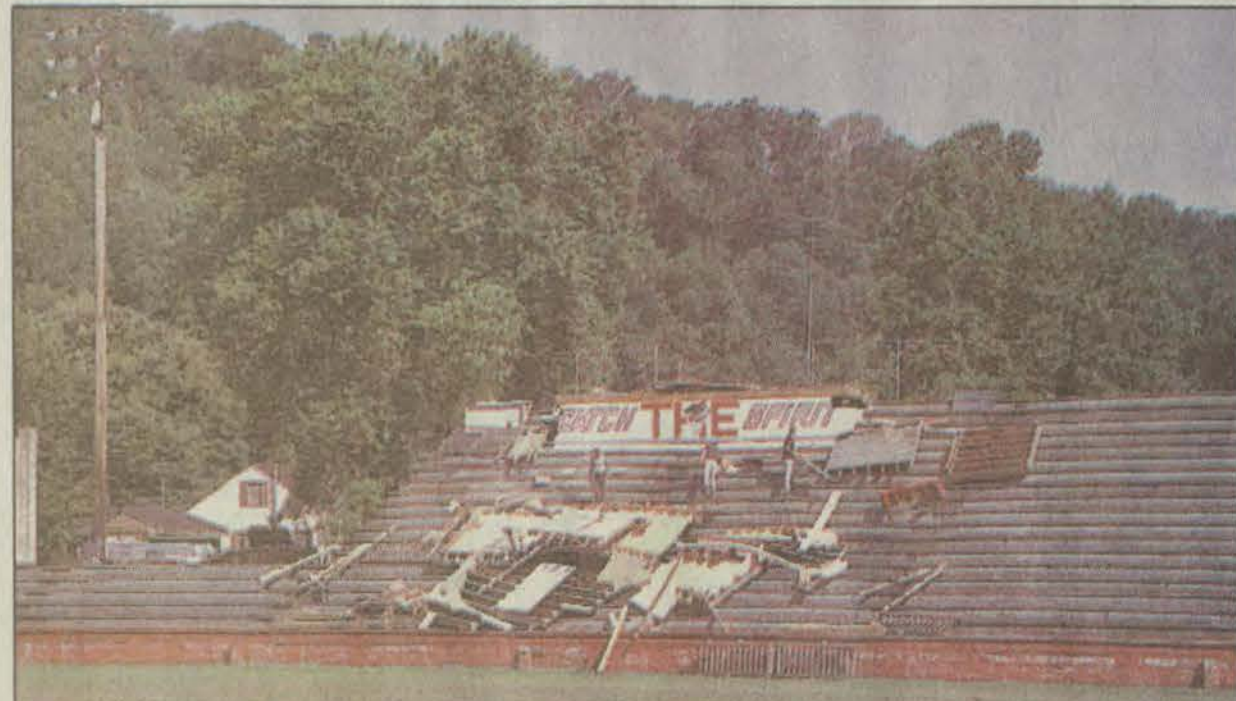
A CREW BRAVED THE HOT SUN as they began to dismantle the old bleachers at the Prestonsburg football field. New bleachers will be moved in for use this football season. The field will undergo renovation after the '99 season. (photo by Ed Taylor)
