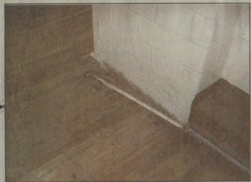
Water seepage over the years has caused deterioration of the flooring in the Prestonsburg Elementary auditorium. The Floyd County Health Department cited the school for a safety hazard because of the condition of the flooring. (photo by Willie Elliott)
