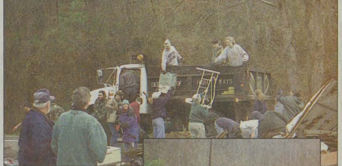
Students on spring break from five colleges helped students of The David School and community members clean up this week along KY 404. They cleared materials from the old school and picked up roadside garbage for road crews to transport to the Garth Hollow transfer station. The group hoped to remove 100 tons of trash from David to the top of David Hill at the Magoffin County line. The volunteers — about 75 in all — are from Notre Dame University in Indiana, St. Ambrose University in Iowa, Edgewood and Viterbo colleges in Wisconsin, and Virginia Tech. (photo by Willie Elliott)
