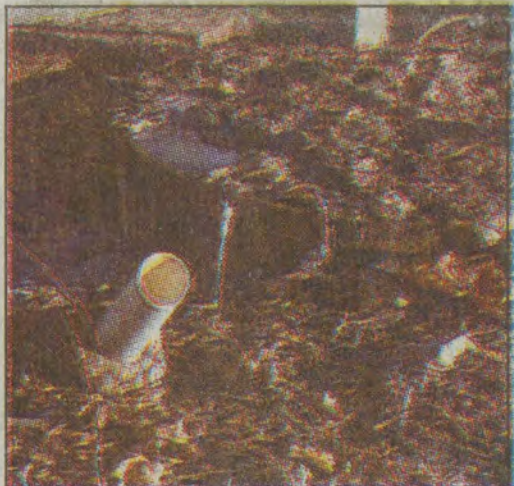
The City of Martin is seeking funds to correct a portion of the water system that leaks sewage on to the ground and then into Beaver Creek. (photo by Willie Elliott)
