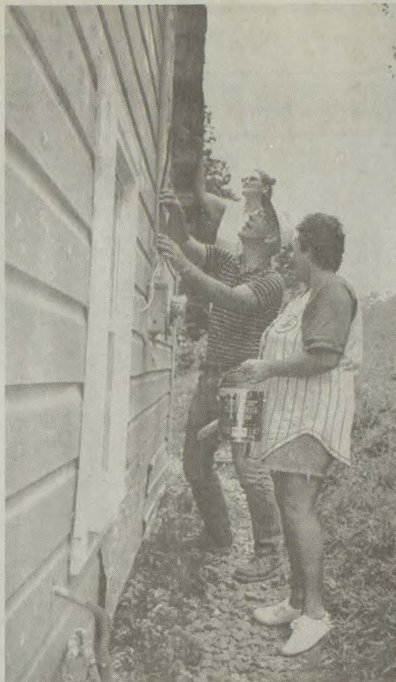
Mary Watkins, homeowner; Father Dick; and Dorothy Vayda applied coats of paint to the Watkins home at Hippo.
