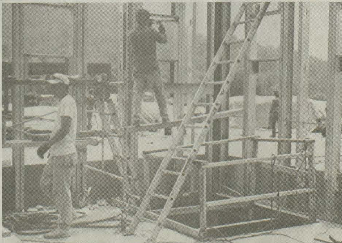
Construction workers continued working this week with the completion of the roof on the new Floyd County Justice Center. The project is slightly behind schedule, a CMW Inc. representative reported to the Floyd County Fiscal Court last Friday, but the contractor anticipates making up time once the roof is finished. The multi-million dollar project is scheduled to be complete in February 1998. (photo by Chris McDavid)
